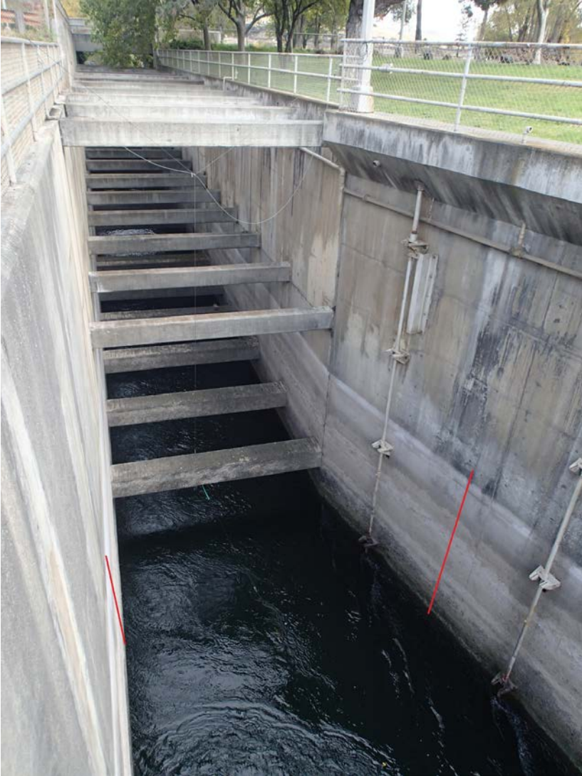
Figure 2. View of proposed location (red lines) of additional antennas in TDA South entrance pool.
